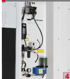
Compress Air and Lubrication System
