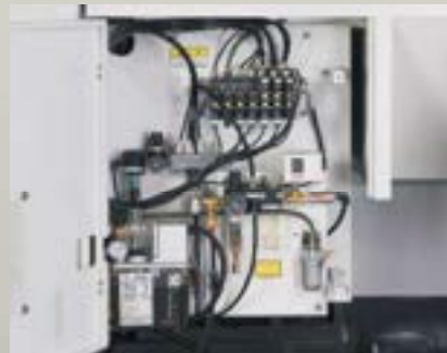
Hydraulic & Lubrication System(LU-620)
