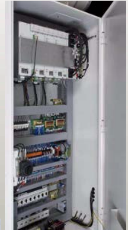
Electric System For Easy Maintenance
